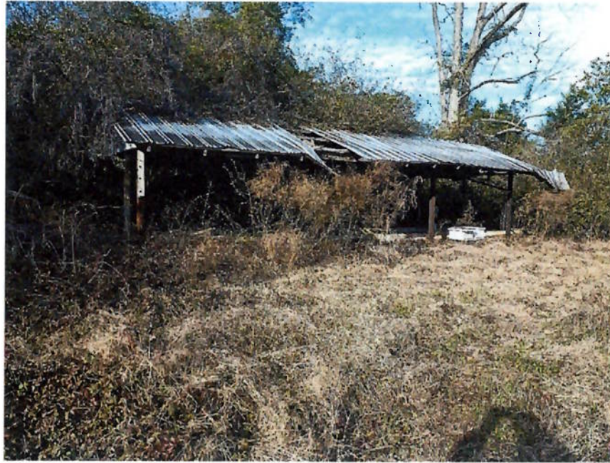
Old Farm Building in Poor Condition
