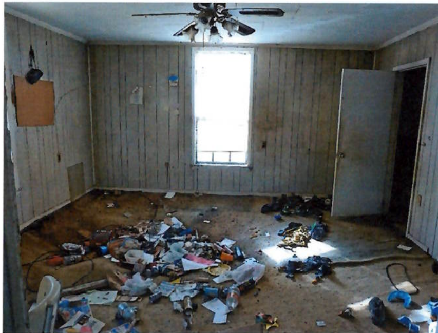
Right Rear Room – Floor Sinking Down
